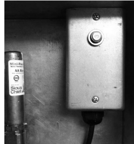
(closed electrical cover)
