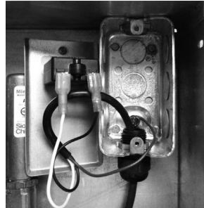
(open electrical cover)
